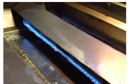
Normal Burner Flames
